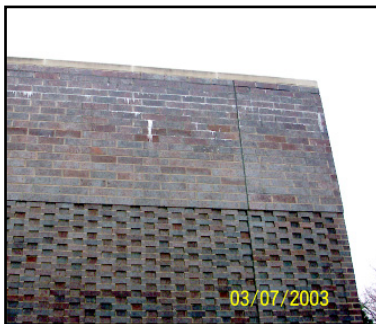
My Bank: (Note the efflorescence, and the flush limestone cap- it should have had 1 1/2" projection, with drip edge and flashing under the cap)
